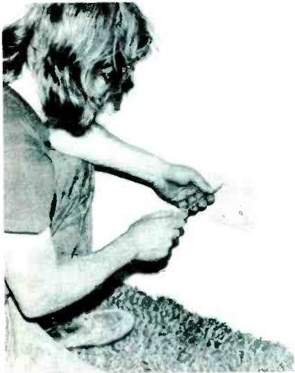
Fig. 11 The installer is finishing a tap-off after the wall has been painted.
